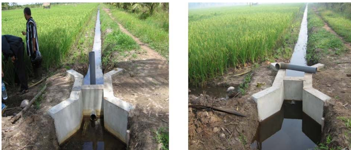
Figure 8 Water distribution structure at the field level
